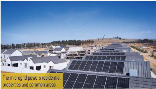
Broadreach and Lesedi installed a network of solar panels and batteries.
